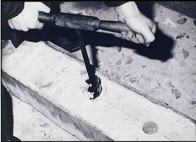
Picture 10. A hand auger is a simple way to drill the two inch holes.
